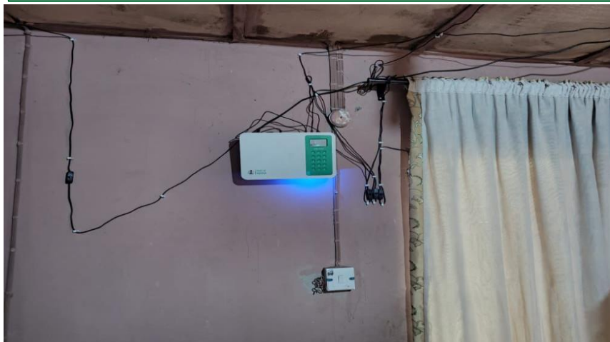
Installed SHS systems
