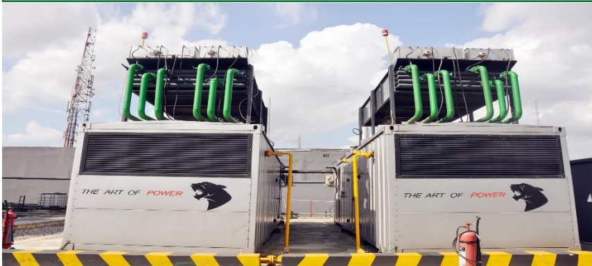
The IPP plant deployed in Ariaria market, Abia State
