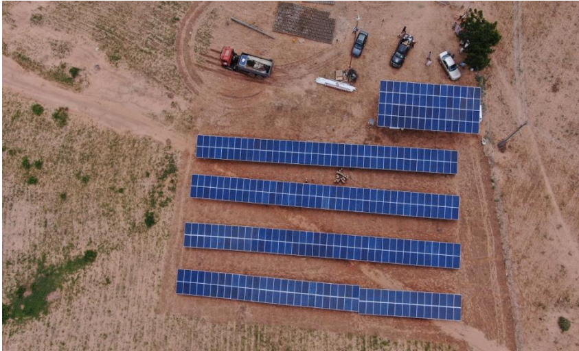
100kWp mini-grid , Eka Awoke Community, Ebonyi State State
