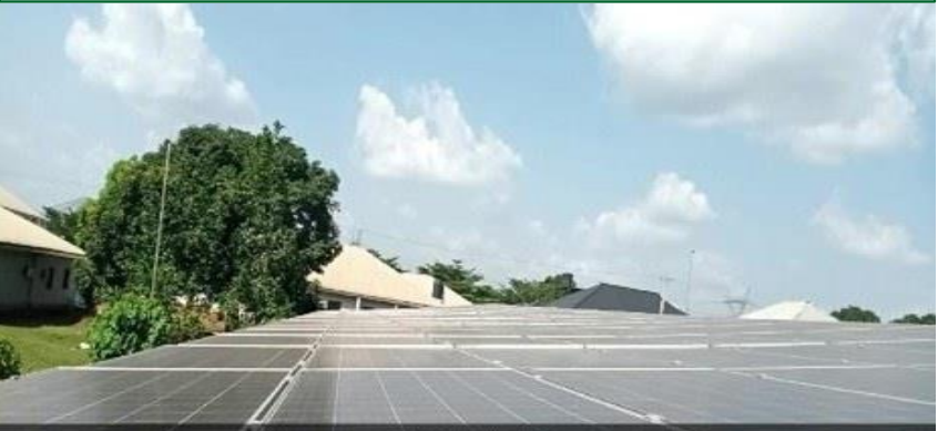
50Kwp containerized system at Irrua Specialist Hospital, Edo State
