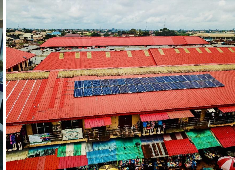
Installed solar PVs powering shops and businesses at the Edaiken market
