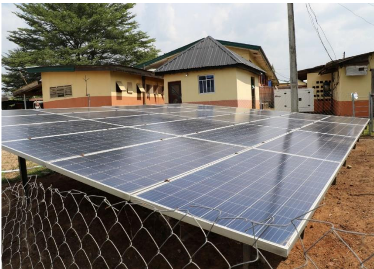
7.5Kwp mini-grid at the Joint Hospital, Ozubulu, Anambra State
