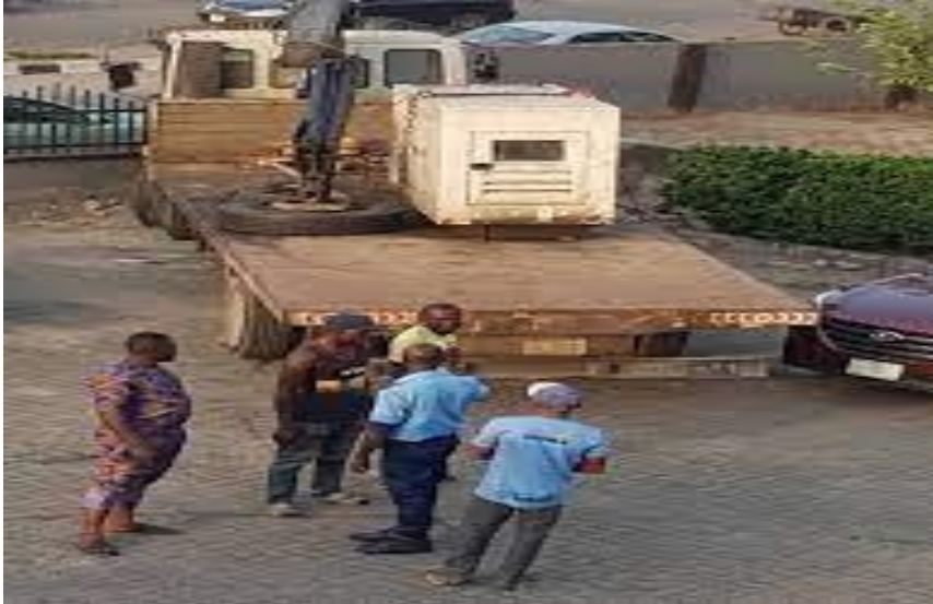
Diesel-powered generating sets being decommissioned at Sura market following the activation of the IPP
